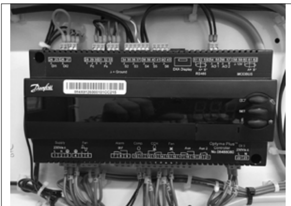
Picture 4 : Normal wiring
