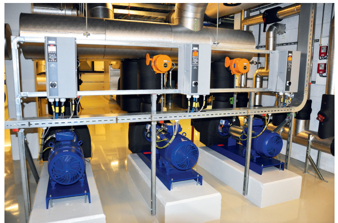
Neat, well-organized installations ensure the best possible up-time.
