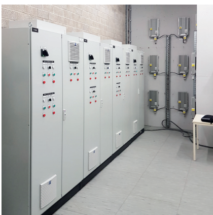
One of the two technical rooms with brake resistors at the end wall.
