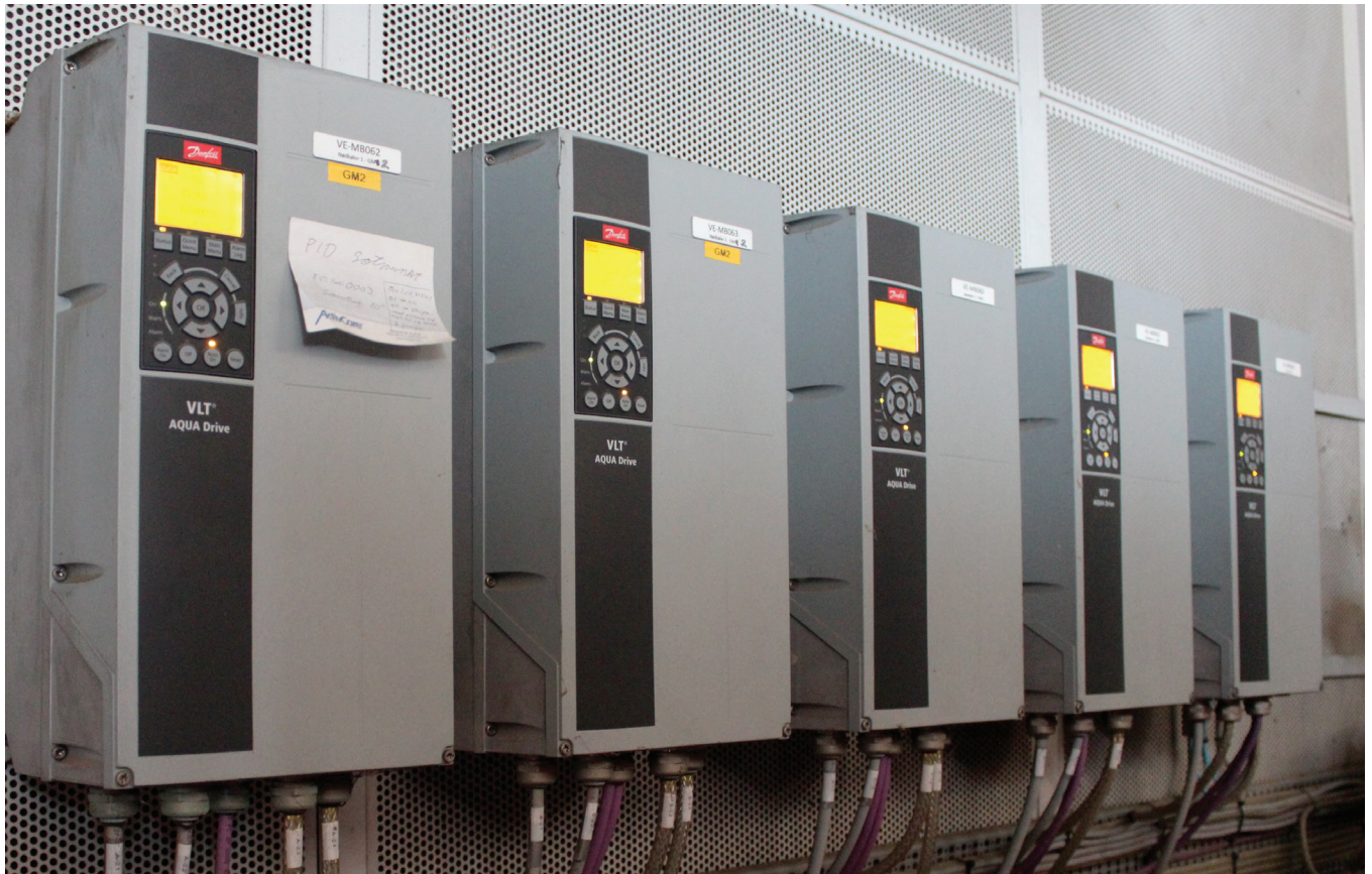
Biogas power generation: VLT® AQUA Drives control cooling fans and booster plant.
