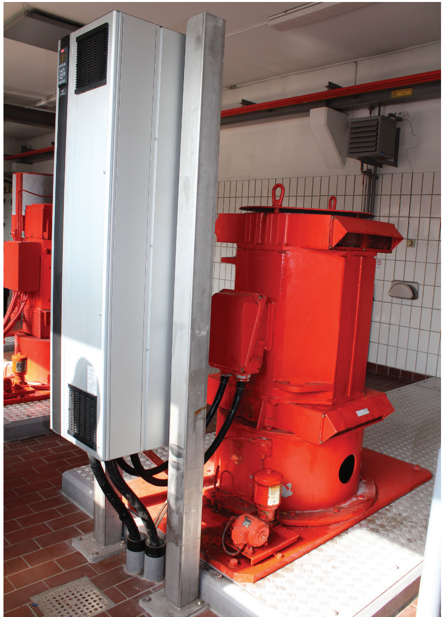
Discharge pumping station: A VLT® rated 160 kW with IP54 enclosure controls this pump weighing 1.25 tonnes
