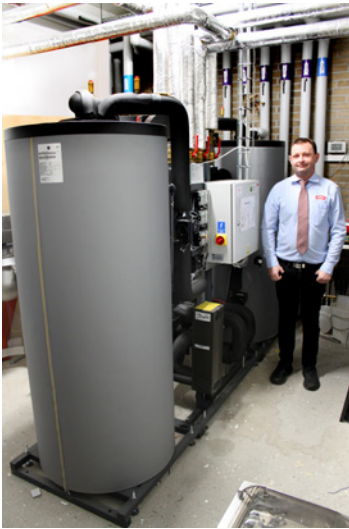
Morten bredvid Heat Recovery Unit (HRU).
