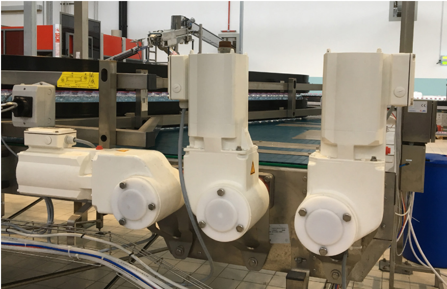
View of the Danfoss VLT® One Gear Drives, installed at the end of the line. IP 69K protection level fulfills requirements for the best hygiene and cleansing design.
