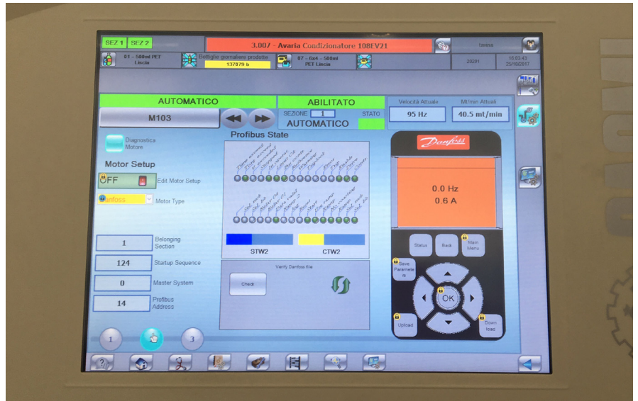
HMI for transporter automation where Sacmi replicated the LCP programming of the frequency converters to potentially modify the parameters of each device without needing to open the electrical cabinet.
