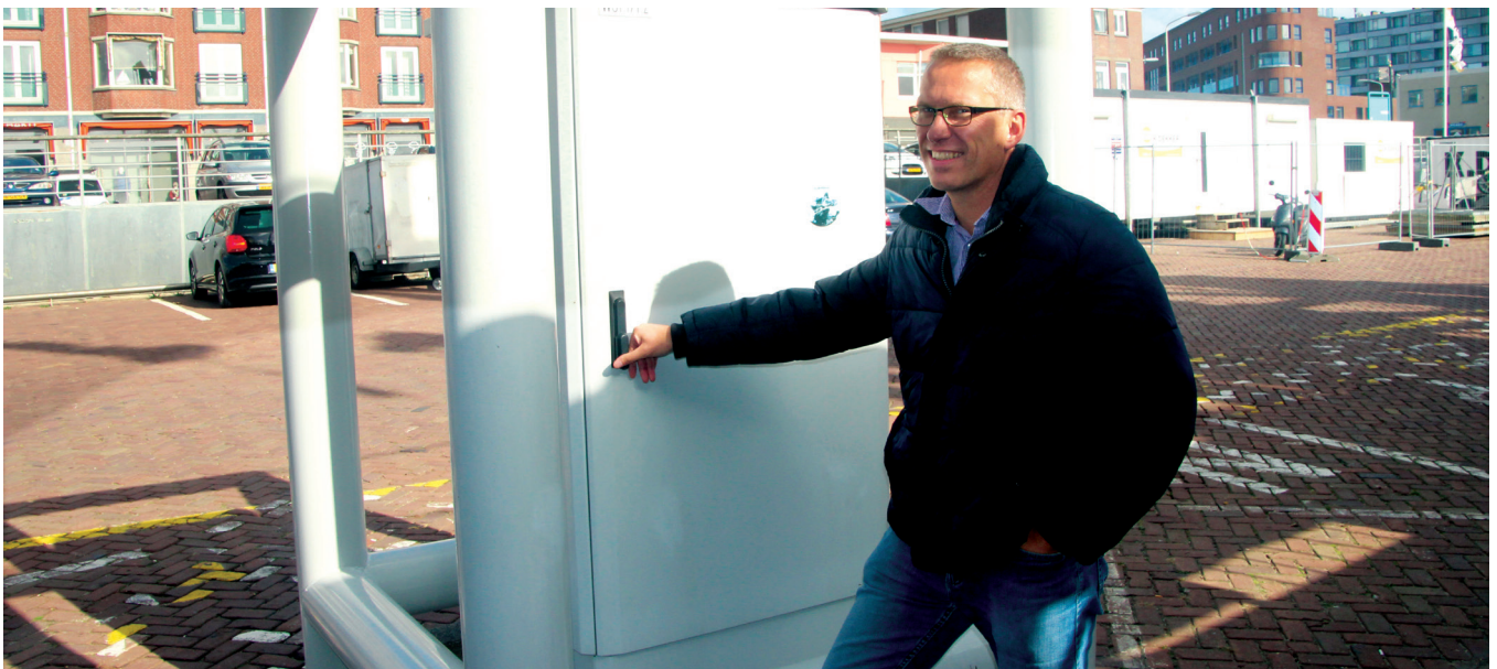
Maarten Hektor demonstrates one of the shore power connection points which are controlled by Involtum's Walstroomb app.
