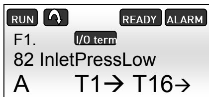
Figure 7.1-4, Low pressure alarm on the NXP panel
