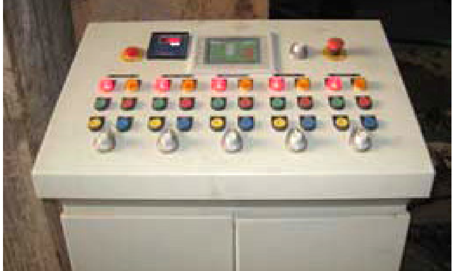
The VIPA Speed7 range of PLC model 315-2AJ10 was selected for its smooth operator interface and for quick response controlling the speed and torque. This has Profibus DP interface, the required number of I/O's and two touch panels.
