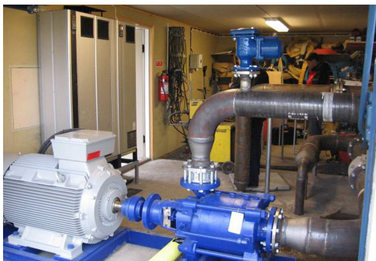
Installed 200kW VLT® AQUA Low Harmonic Drive controlling a new feed pump and maintaining a constant flow of water through the hundreds of meters of pipes
