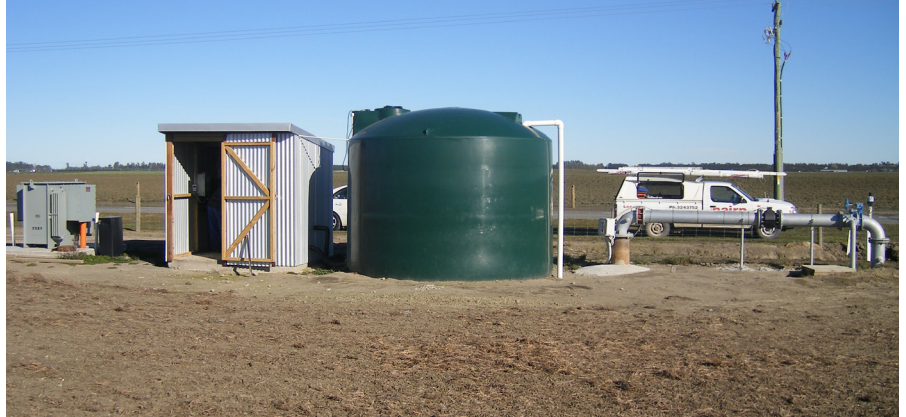
A 160kW VLT® AQUA Low Harmonic Drive installed on a submersible pump in Rakaia, in central Canterbury, New Zealand.
