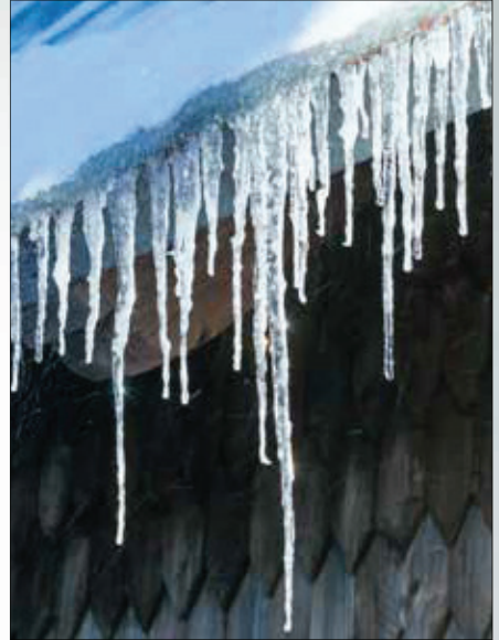
RX Roof & Gutter De-Icing
