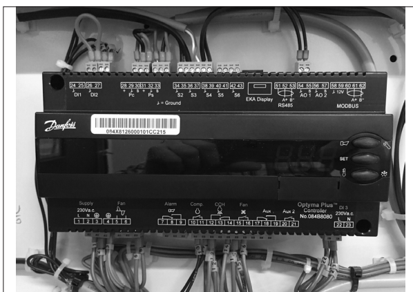
Picture 4 : Normal wiring
