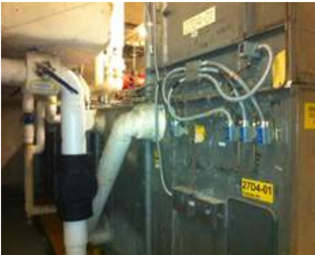
Underperforming central station AHU
