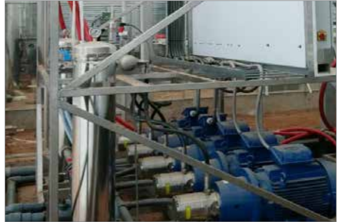
Five Danfoss PAHT 90 pumps help to provide pressure for the misting system.
