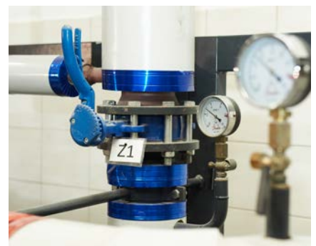
District heating system fixtures
