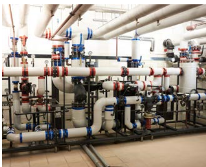
DSE large heating substation in building "O"
