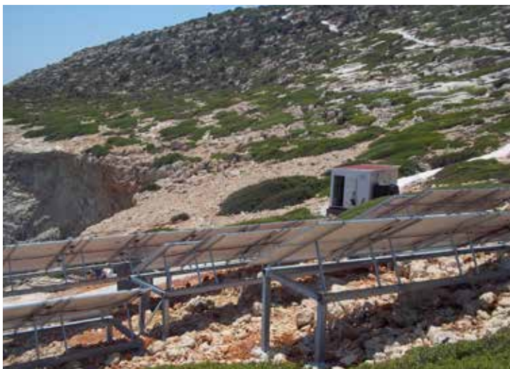
Solar-powered SWRO plant located on Stronglli
