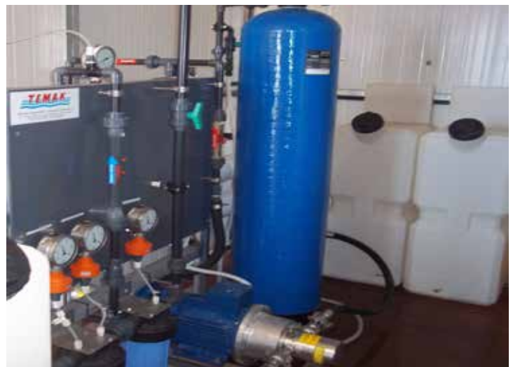
The SWRO system with a Danfoss APP 3.5 pump and APM 2.5 ERD
