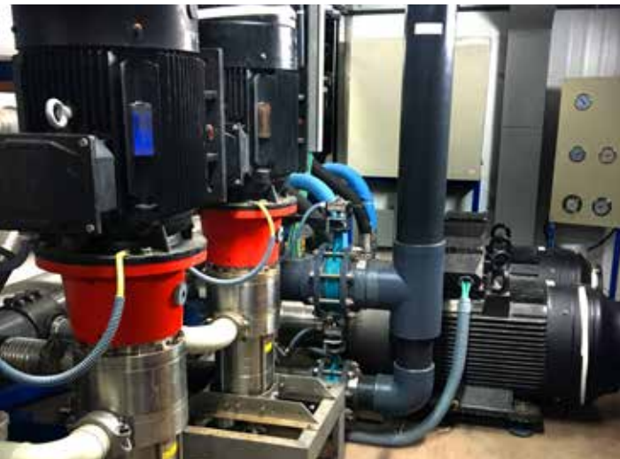
The containerized solution with APP 38 pumps and iSave 50 ERDs
