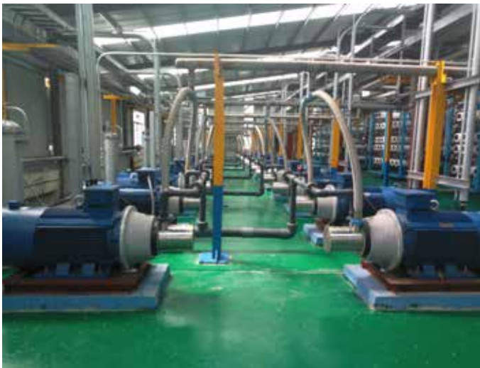
Danfoss APP W 24 pumps operating in parallel
