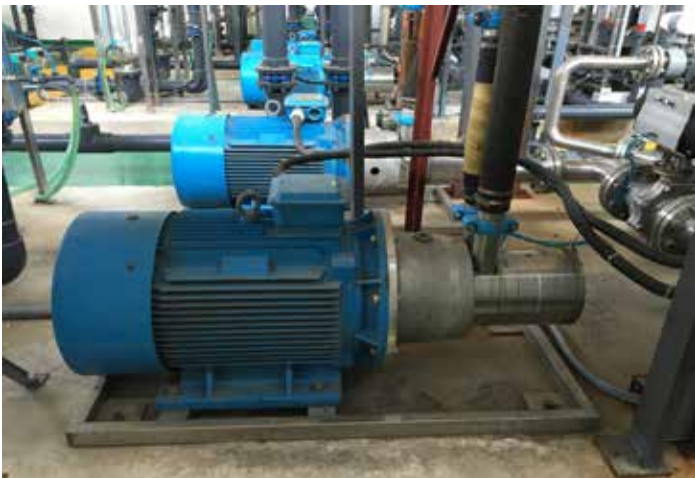
RO plant with two trains - each using two APP 30 pumps
