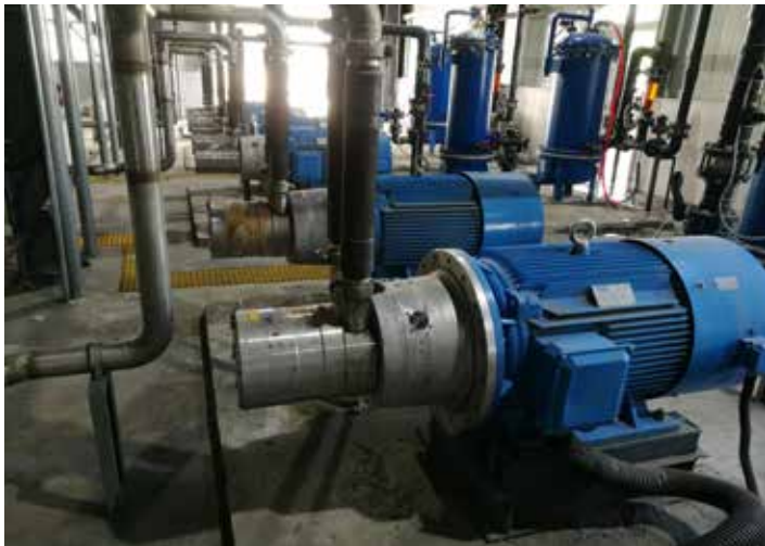
Danfoss APP pumps operating in different trains at Chuan Ning Biologicals ZLD treatment plant
