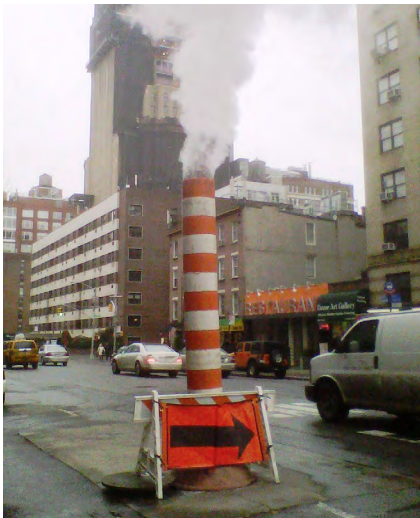
FIGURE 3: A chimney for dispersion of condensation from the steam distribution network. The condensation can be caused by water coming into contact with the steam pipes being boiled or leakage of the steam pipes.
