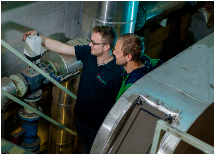
Both the heating plant and the customers use Danfoss products.
