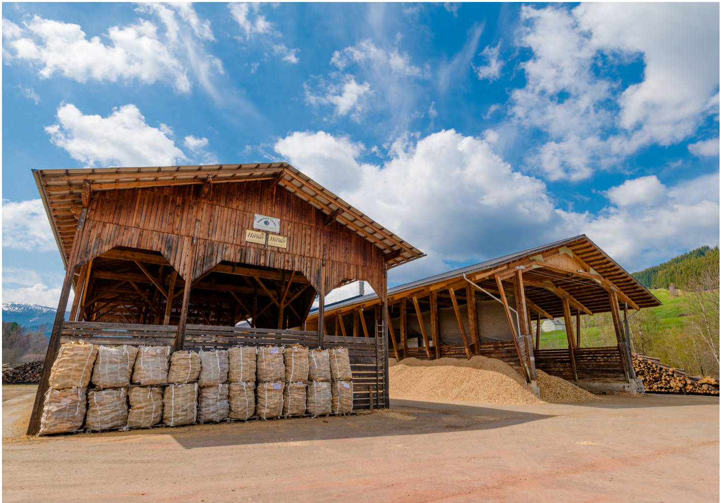
Biomass directly from the region: In the heating plant, two boilers with 1 or 2.2 MW of combined heat and power supply ensure reliable district heating for the approximately 150 customers in St. Lambrecht.
