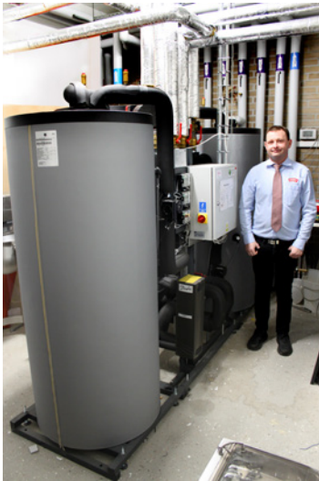
Morten at the Heat Recovery Unit (HRU).
