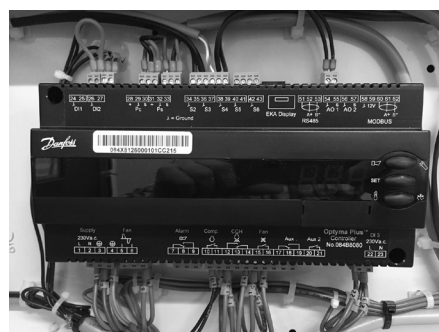
Picture 3 : Normal wiring
