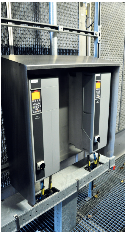
Outdoor installation for the regulation of the cooling towers, comprises two VLT® HVAC Drive FC 102 drives in IP55 enclosures, with built-in disconnect switch.
