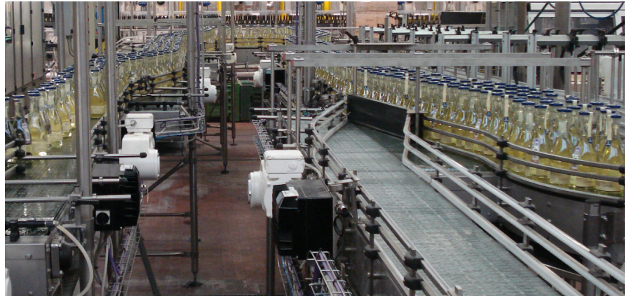
Bottling line with VLT® OneGearDrive® and VLT® Decentral Drive FCD 302 installed directly on the conveyor
