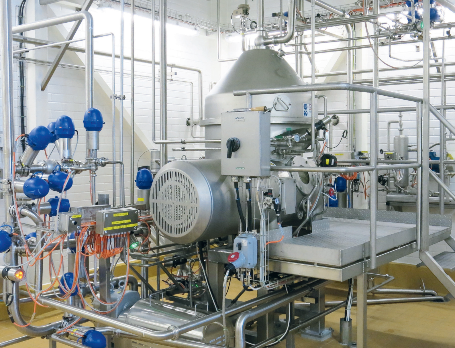
Valio's Seinäjoki plant produces all Valio quarks. A separator is used for producing quark. The pumps and mixers used by the separator are controlled by VACON® 100 AC drives. In recent years, quarks have been the quickest-growing product category in retail sales. Valio was able to quickly double its production at the Seinäjoki plant as butter production had recently moved to new premises.
