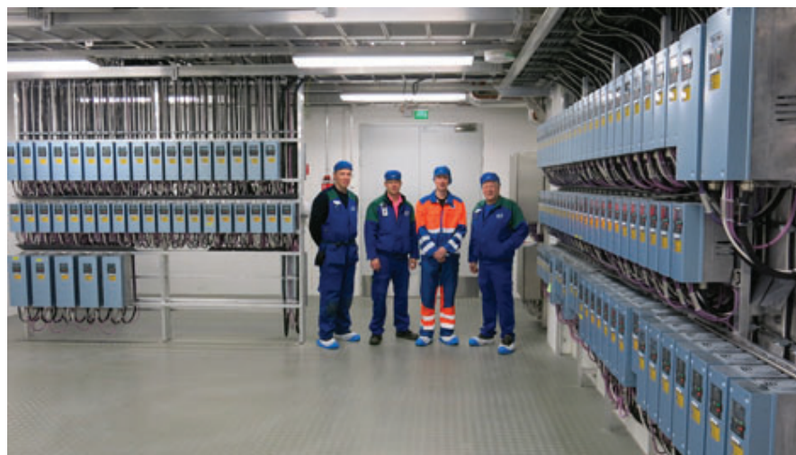
All VACON® AC drives delivered to the Seinäjoki plant are provided in splash-proof IP54 enclosures. Hannu Teräväinen (front left), Pauli Parvi, Teemu Takala (back left) and Marko Vähäkoski inspecting one of the electrical rooms.
