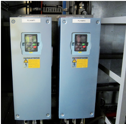
Drives for cooling water pumps
