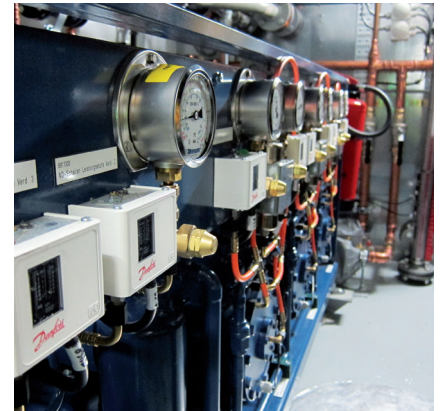
Also the refrigeration system is controlled by Danfoss components
