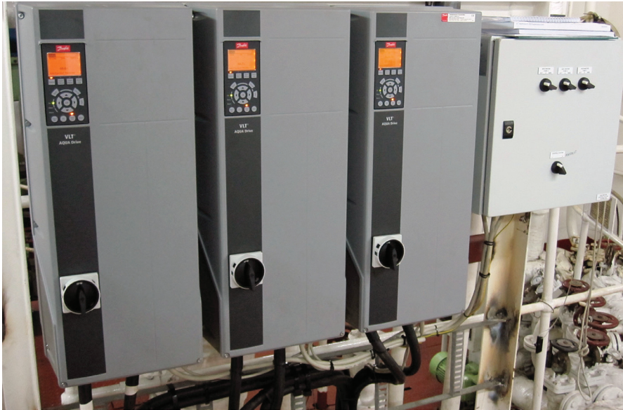
The solution at Dampskibsselskabet NORDEN A/S consists of 3 VLT® AQUA Drive FC 202, 45 kW frequency converters with a cascade pump controller, an electrical switch box for control, and two temperature transmitters.
