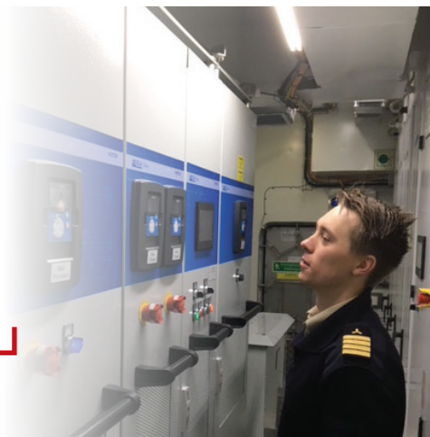
VACON® drives power the main propulsion and thrusters
