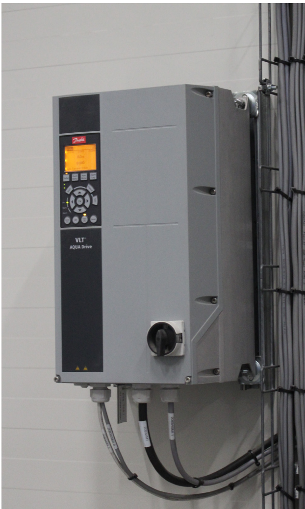
VLT® AQUA Drive FC 202 controls pumps and blowers at the large biogas plant.
