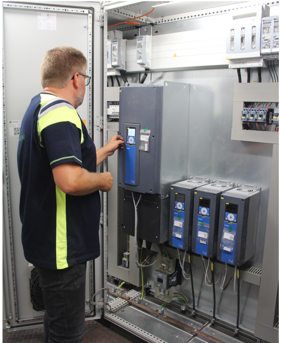
Danfoss Drives' VACON® 100 was supplied by Bilfinger directly from Germany, mounted in a container, ready for use when the plant was commissioned in April 2018.
