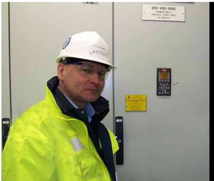
Paul McLaren, E&I Engineer for Ensus, in front of a control panel with 315 kW VLT® High Power Drive and VLT® Advanced Harmonic Filter.
