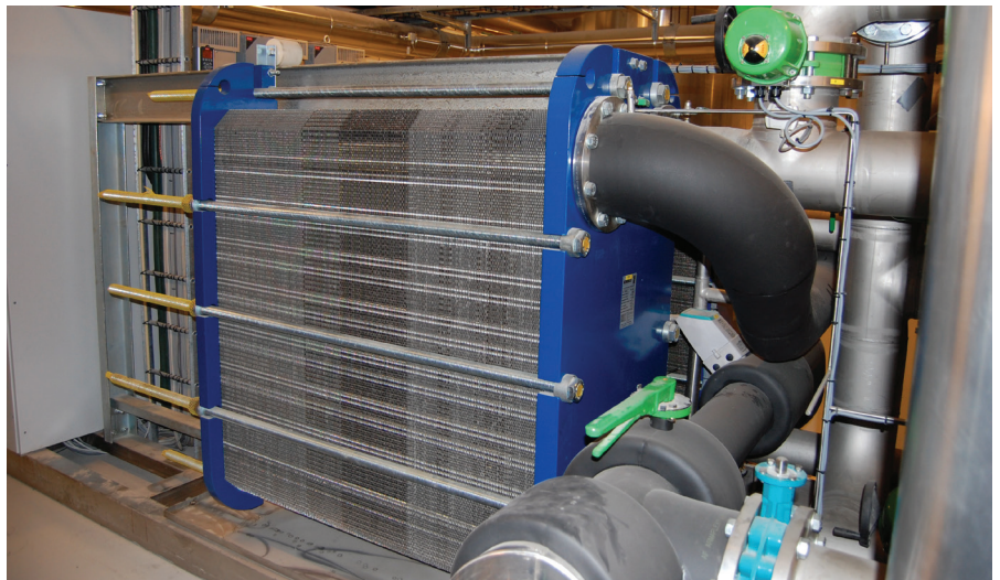
The cooled water from the heat exchanger is circulated in the building to cool rooms to the desired temperature. No active refrigeration is required.
