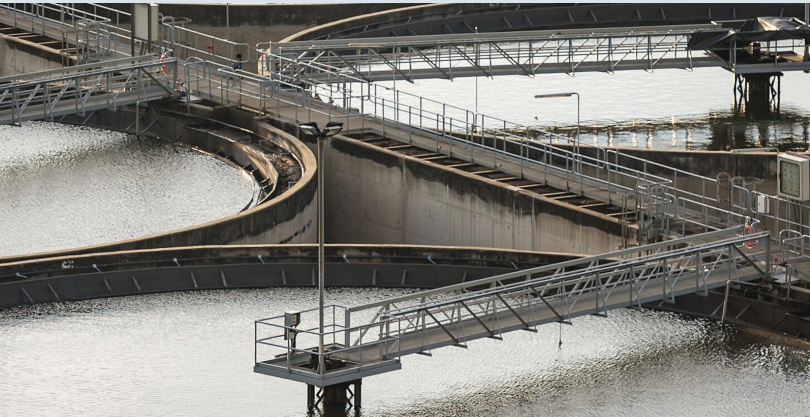
At Putrajaya Sewage Treatment Plant, active harmonic filters keeps the THVD below 5%.
