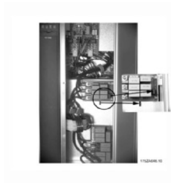
Position of RFI switches
