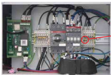
Jumper on slots CNB41 and 43 bridge the digital input DI2. Condensing unit is in pressure control mode.
