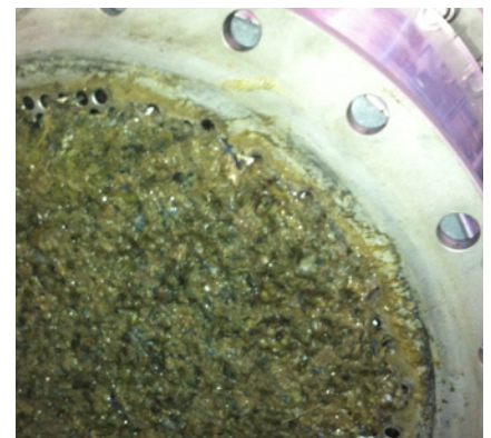
Clogged turbular heat exchanger that requires cleaning.
