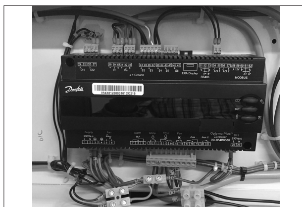
Picture 5 : Temporary wiring
