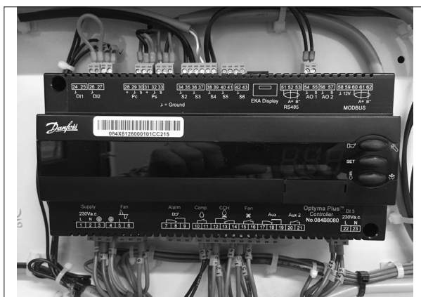
Picture 4 : Normal wiring
