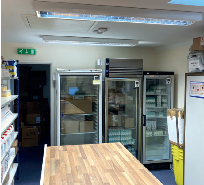
Before, the medicines were stored in nine standalone refrigeration cabinets.
