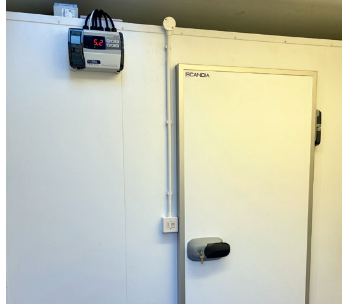
Establishing the connected cold room, the Vet practise can now rely on remote monitoring and alarms to secure stable and optimal temperatures at all times.
