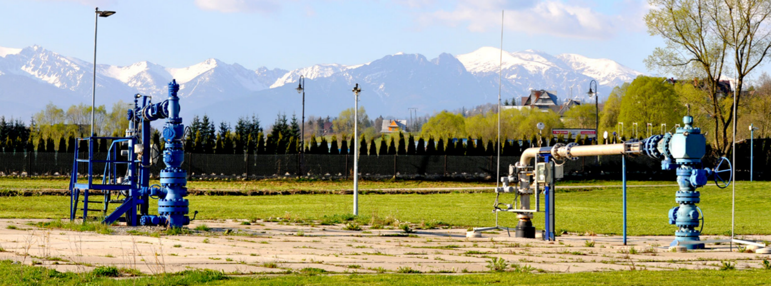
Geotermia Podhalańska, harnesses an impressive 98.89% of geothermal resources for heating homes and generating hot water.
