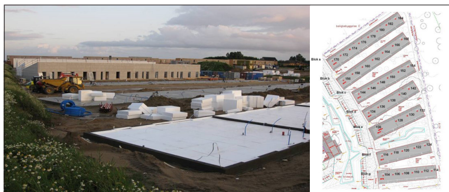
FIGURE 1: Low-temperature DH supply for an area in Lystrup/Denmark. Construction site and area plan
