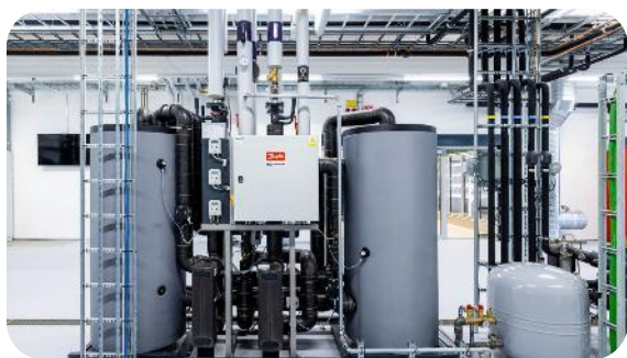
Heat Recovery Units
