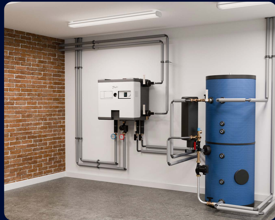
Centralized heating and domestic hot water systems
