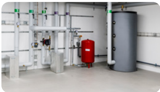
Warm tapwater boilers
