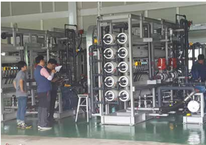
Two trains built around two APP 26 and two iSave 21
